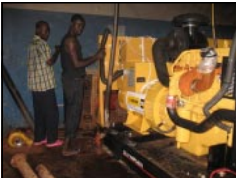
The new generator being installed. Thanks to the Dicken's family for their generous contribution, filling an important need for BMC.
